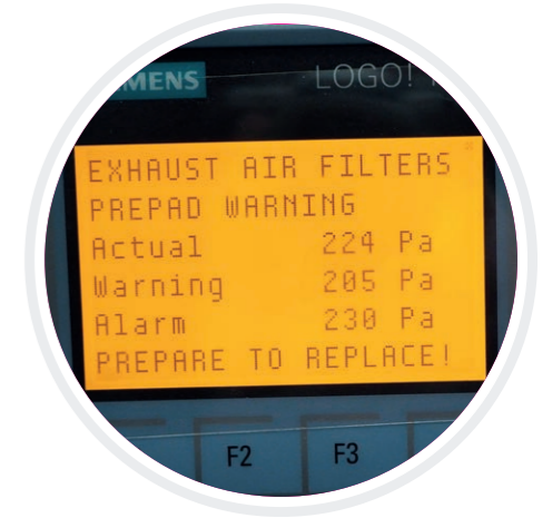
Integrated PLC Control System
