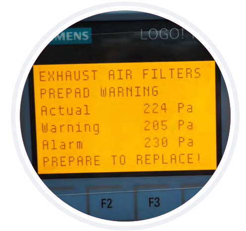
Integrated PLC Control System
